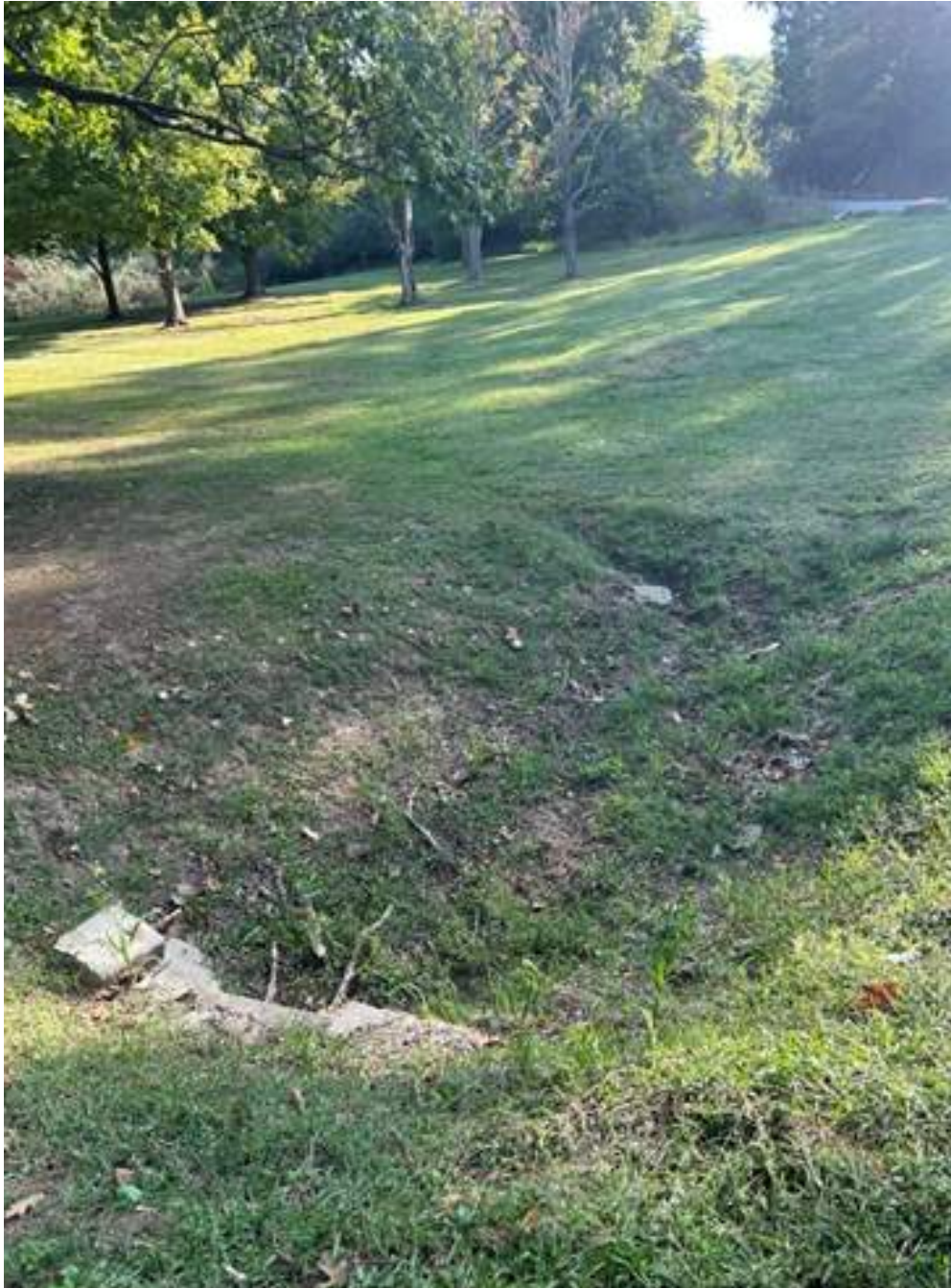
Erosion present at the culvert going under Crayfish Drive. Kurn Road is in the upper right corner of the photo.
