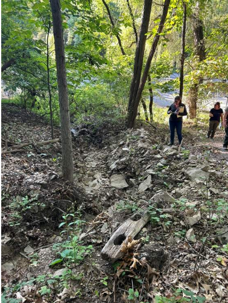
Substantial erosion on the slope between the Blue Gill Shelter and the parking lot. Check dams would slow and retain any runoff not managed by the introduction of the rain garden, berm, and retentive grading above.
