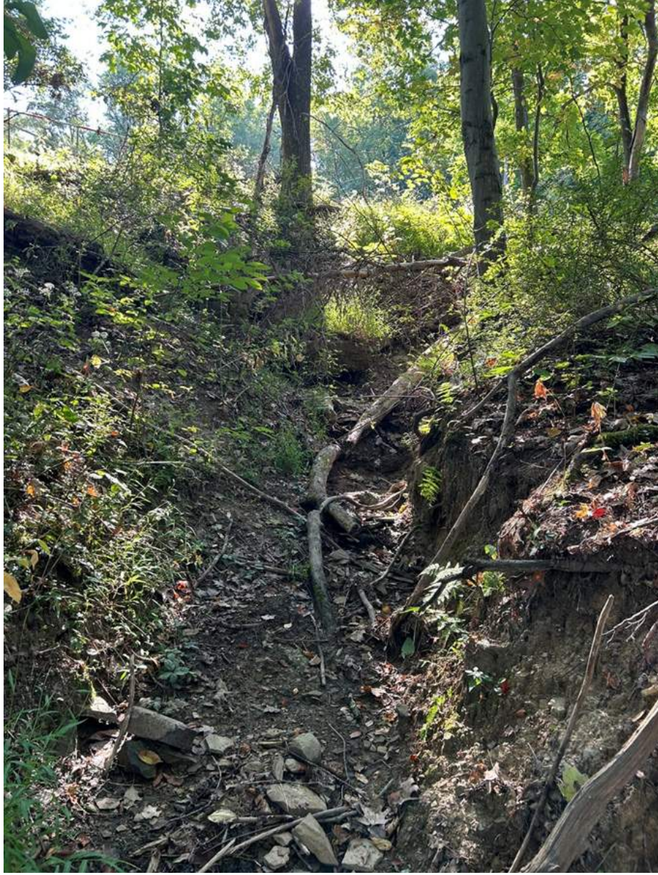
Significant erosion from stormwater runoff in the wooded area below Crayfish Drive.
