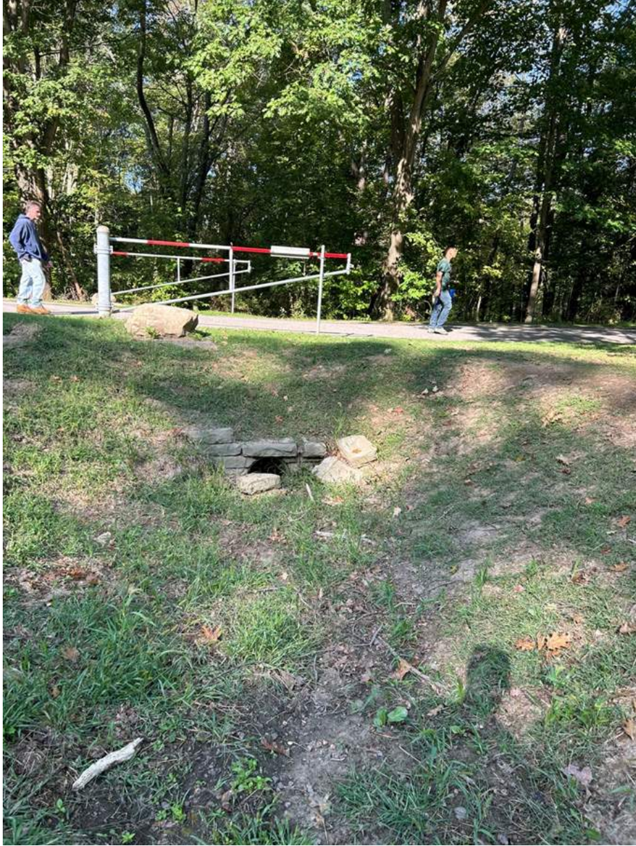
Erosion at the culvert under Crayfish Drive, with the wooded area beyond.
